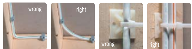
Don't bend the cable; instead, create a smooth, gradual curve. Plastic wire ties should be snug, but not tight enough to pinch the cable.
