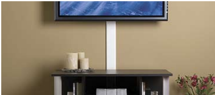
One easy way to hide the wires between your wall-mounted TV and A/V cabinet is to use décor-friendly cable management raceways.
